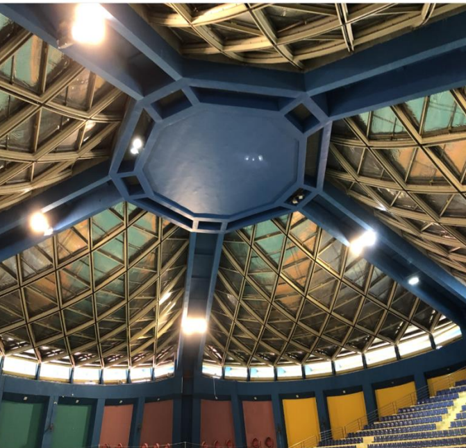
Woodland Sports Hall Roof
